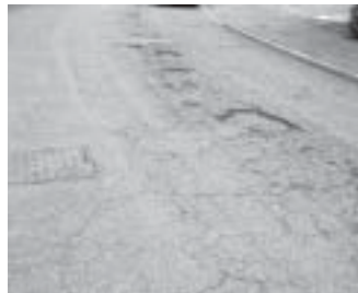
Poor road surfaces
