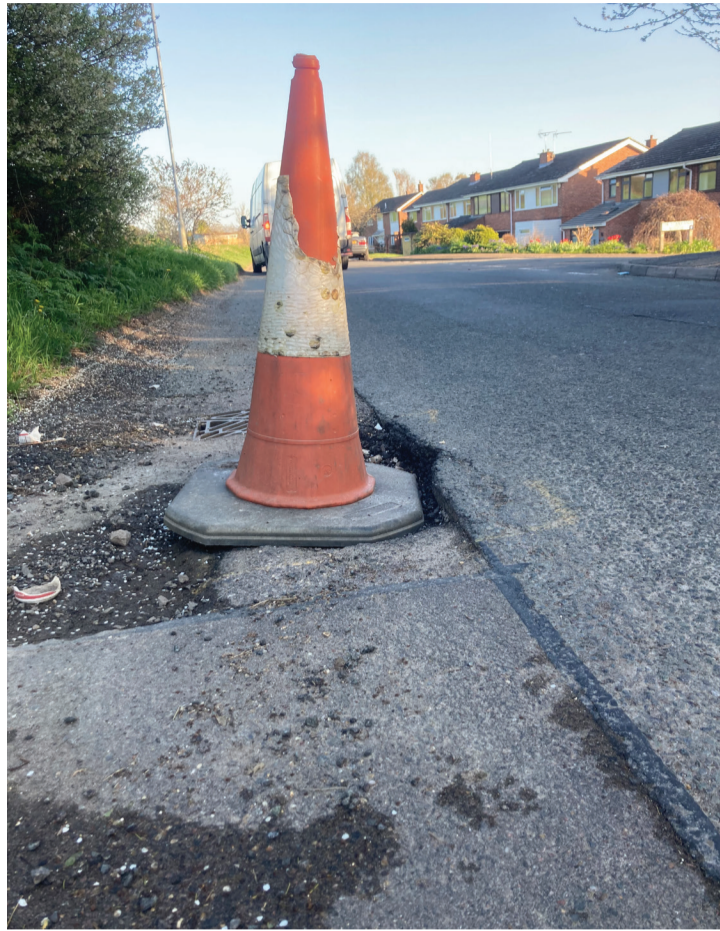
Linton has been plagued by potholes in recent months
